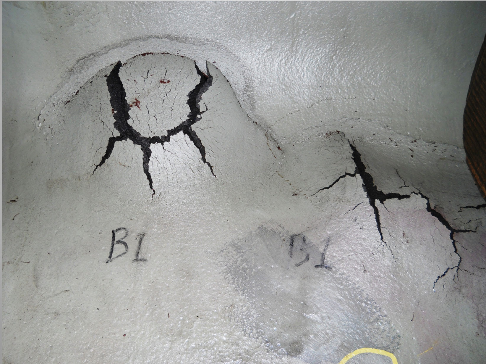
Damaged B1 Cam box
