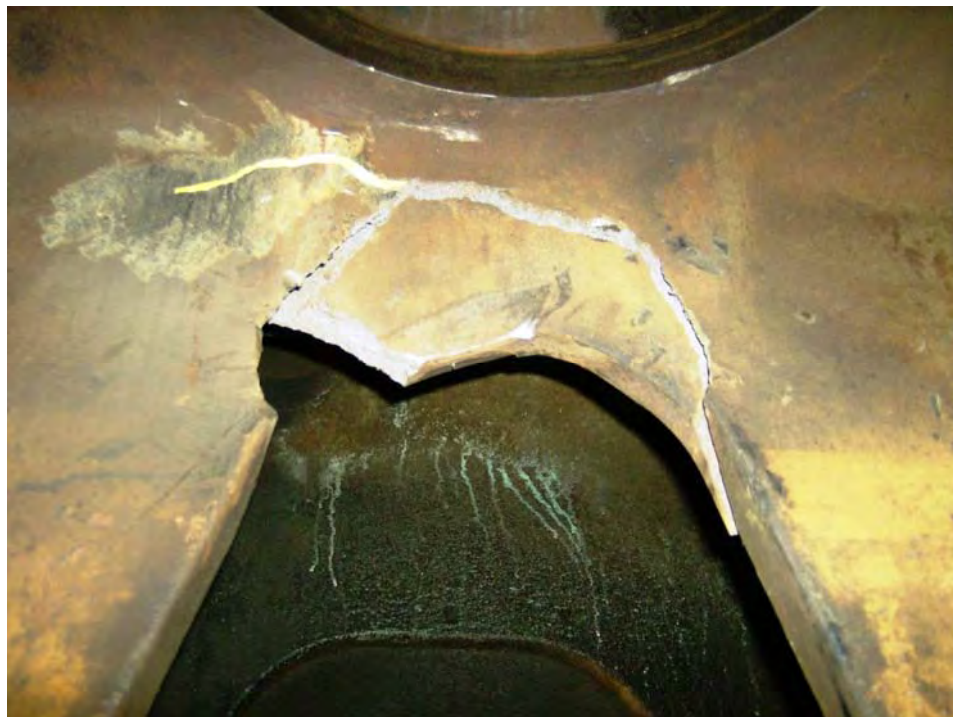
Scavenging trunk damage
